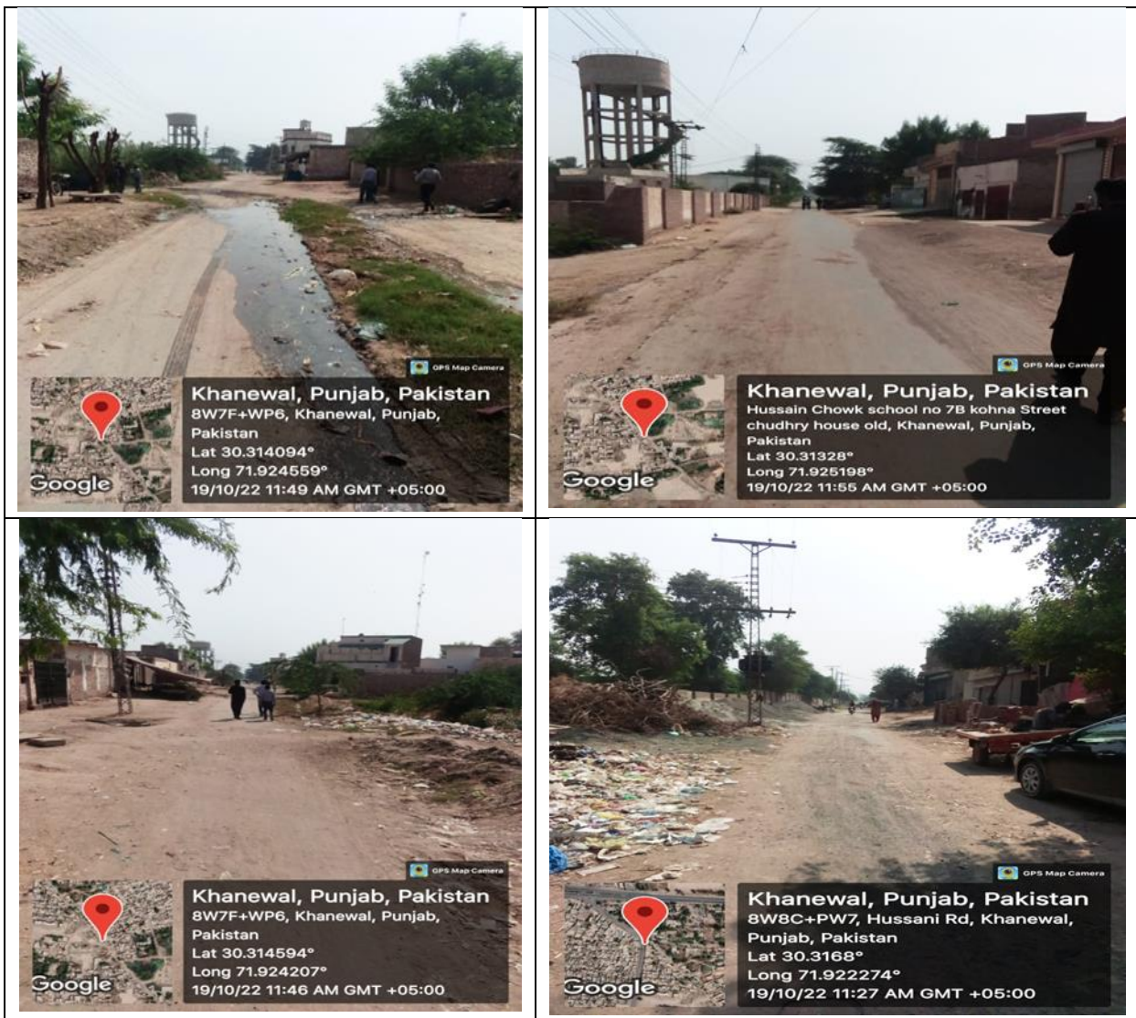
Figure 1: A view of deteriorated condition of Old Karkhana Road
