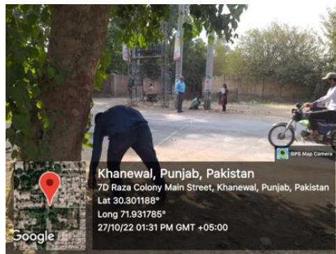
Figure 26: The poles that will be shifted are the ones for avoiding the tree cutting
