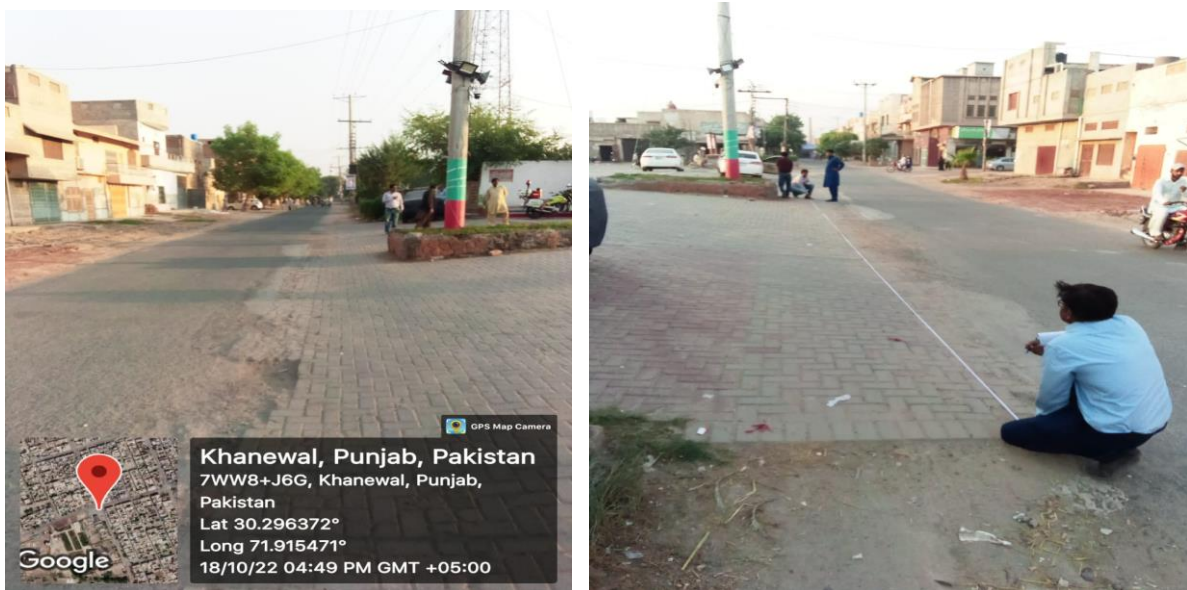
Fig 4-1: Tough Paver outside the petrol pump which will be restored by the contractor after construction work of new water supply line
